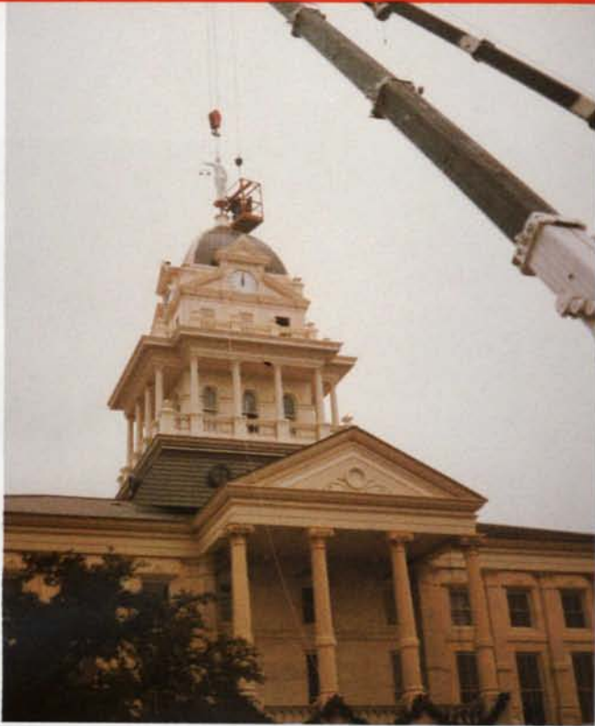
Reproduction And Installation Of Historic Cupola Bell County Courthouse The Williams Company, AIA Belton, TX. Austin, TX. ....Cupola 39' Wide x 58' High....
